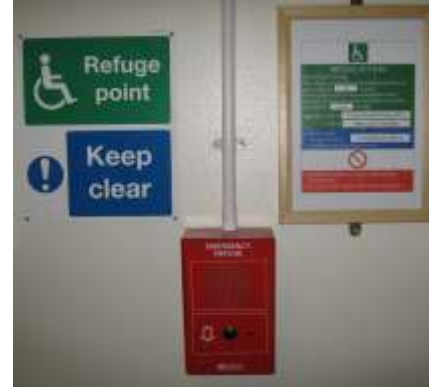
Fire refuge with signage and communication system
