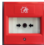
Fire alarm call point
