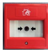
Fire alarm call point
